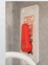
Hot water bypass valve
